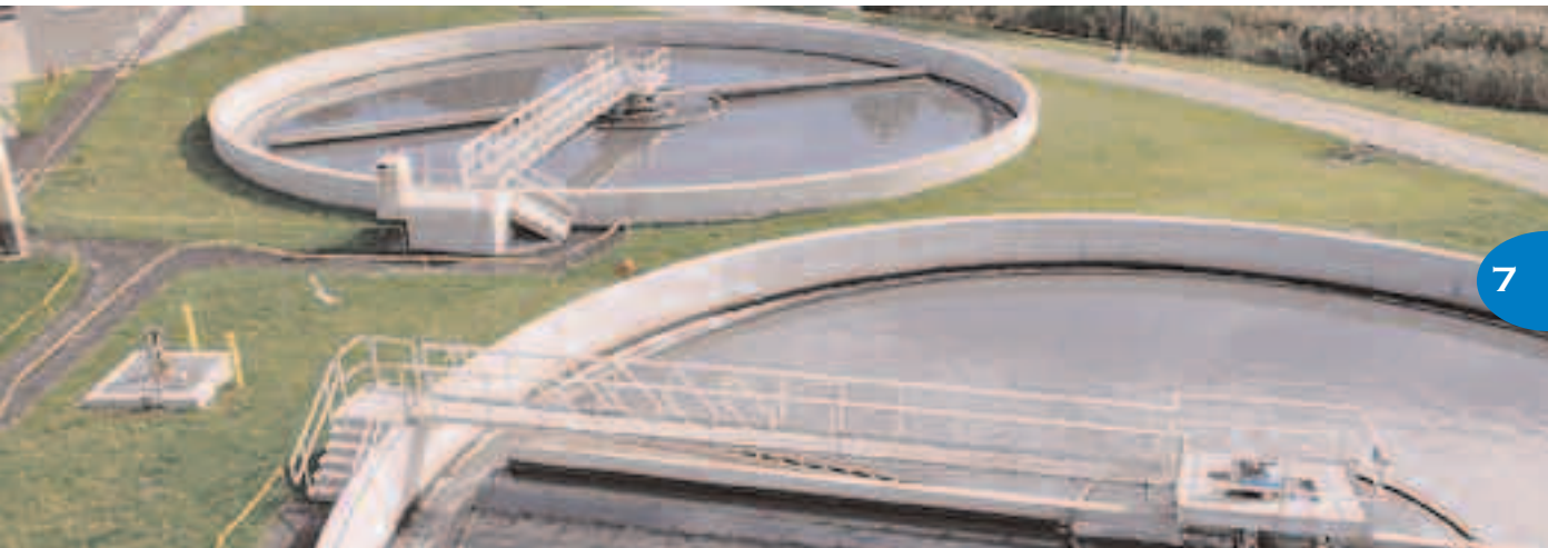
NBC-BUCKLIN POINT WWTF CLARIFIERS
